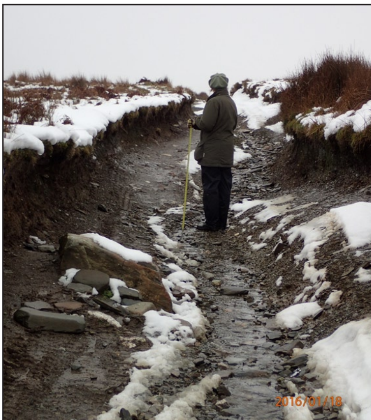
Visible deep erosion on the Whitestones route (photo: Save our Paths)
